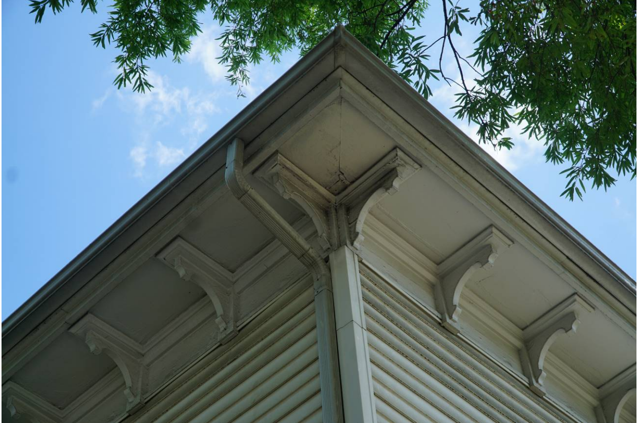
Photo 10: 741 South Main Street, Harrisonburg, VA. South Elevation, view to northeast. 14 July 2021. Detail of cornice.
