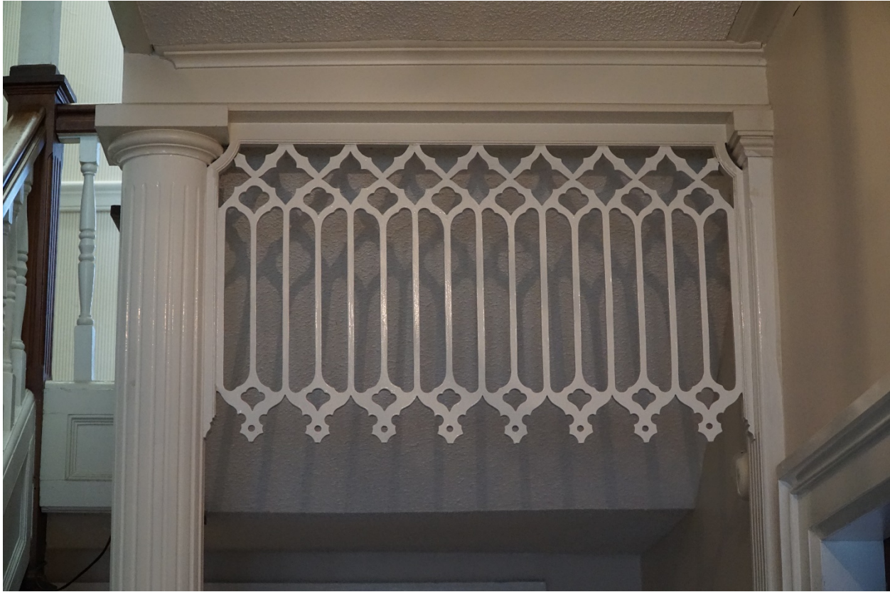
Photo 22: 741 South Main Street, Harrisonburg, VA. First Floor, center hall, view to west. 14 July 2021. Detail of hall screen.
