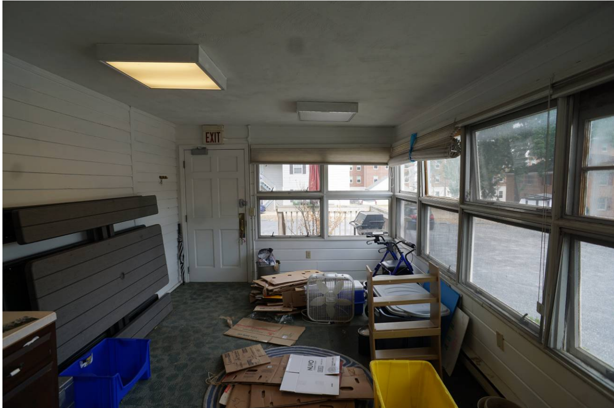
Photo 35: 741 South Main Street, Harrisonburg, VA. First Floor, enclosed rear porch (ell), view to west. 14 July 2021.
