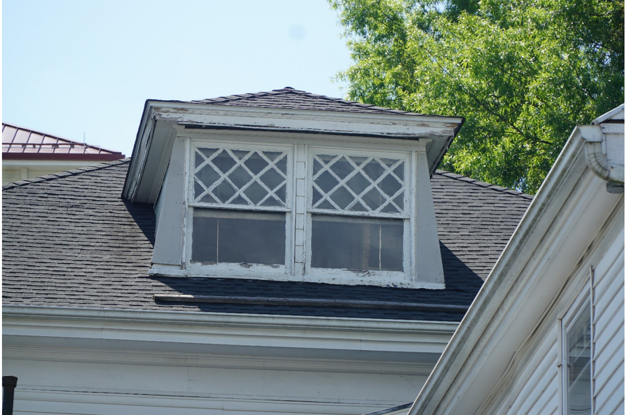
Photo 12: 741 South Main Street, Harrisonburg, VA. West Elevation, view to east. 14 July 2021. Detail of dormer.
