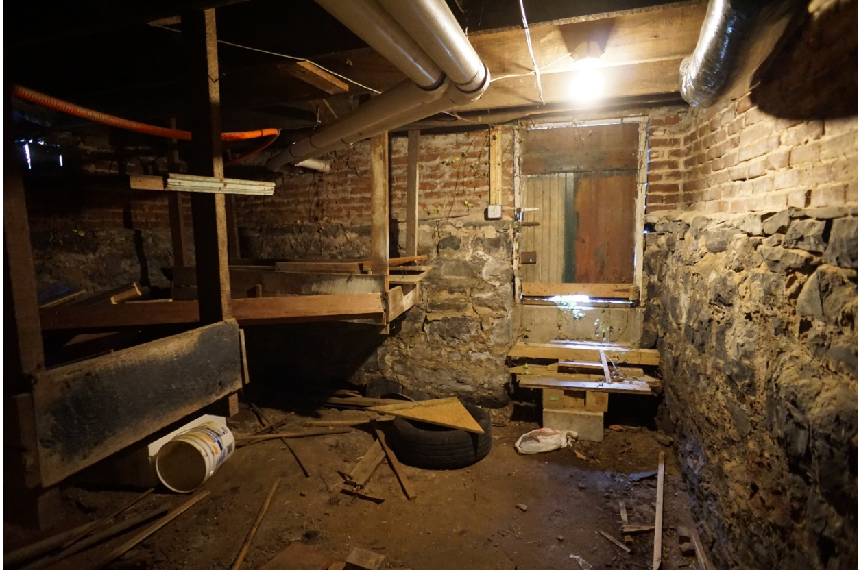
Photo 20: 741 South Main Street, Harrisonburg, VA. Basement (under ell), view to west. 14 July 2021.
