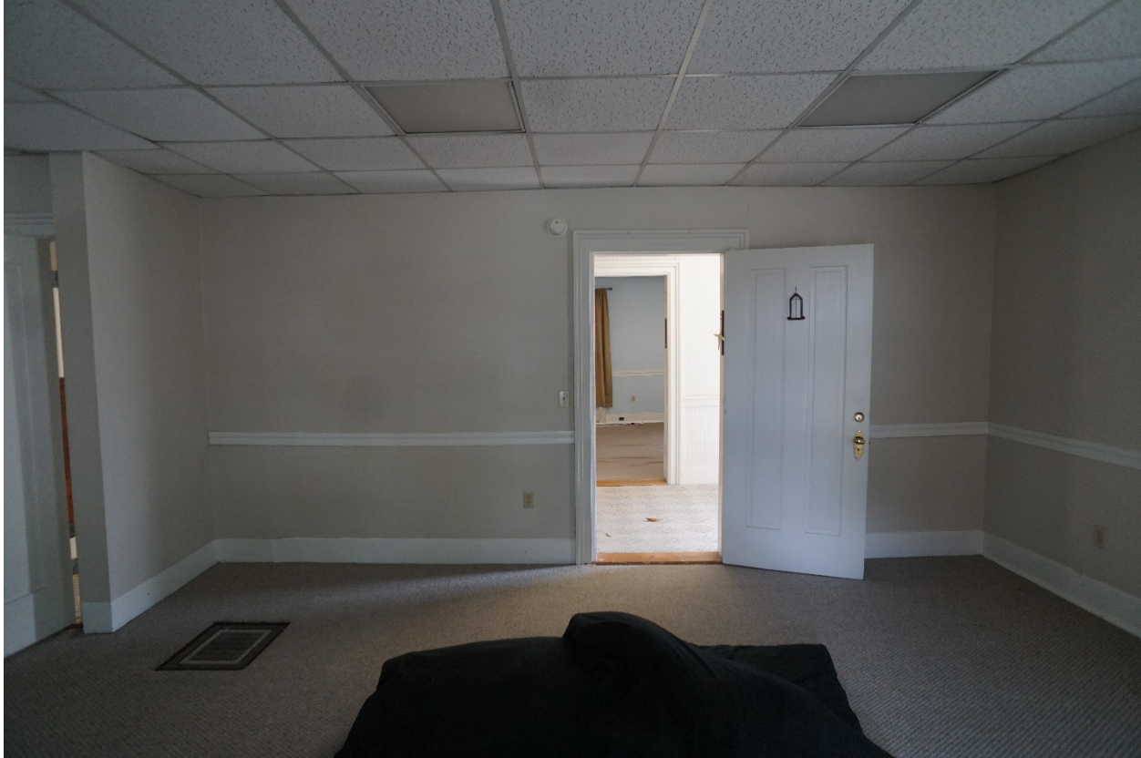
Photo 43: 741 South Main Street, Harrisonburg, VA. Second Floor, SE room, view to north. 14 July 2021.
