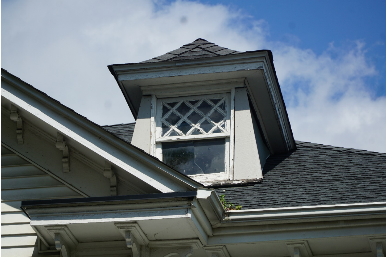
Photo 6: 741 South Main Street, Harrisonburg, VA. East Elevation (primary), view to west. 14 July 2021. Detail of window over entry portico.
