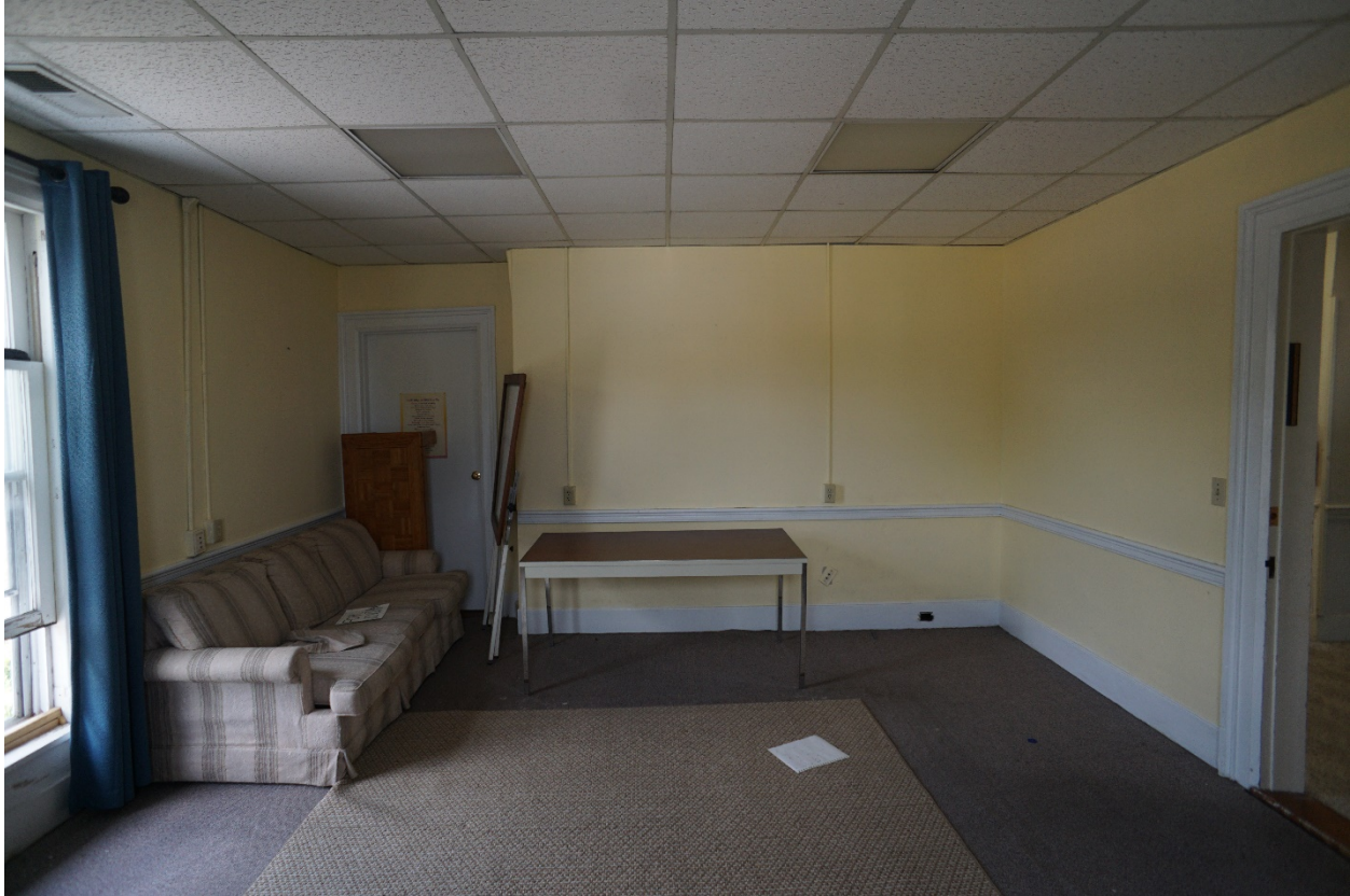
Photo 41: 741 South Main Street, Harrisonburg, VA. Second Floor, NW room, view to east. 14 July 2021.
